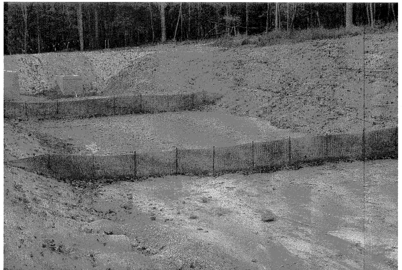
FIGURE 6.65D EXAMPLE OF POROUS BAFFLES MADE OF 700 GPM COIR EROSION BLANKET AS VIEWED FROM THE INLET
