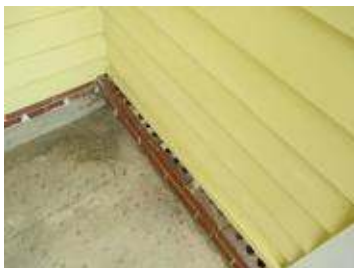
There is a fair amount of paint on brick or surfaces it shouldn't be from a previous painting project.
