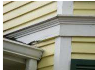
This proposal includes repair to the fascia on the left side of the front bay window.
