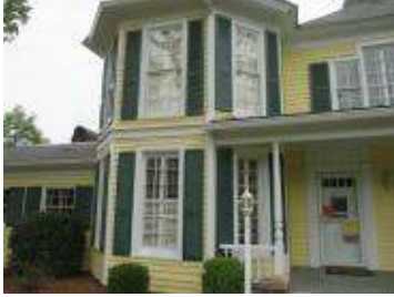
Painting to the specified exterior surfaces of the Weddington Town Hall and garage in a matching color and sheen.
