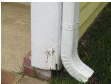
This proposal includes repair to the bottom of the right front corner board of the garage.
