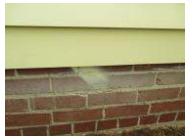
There is a significant amount of paint over spray on the brick, particularly in the back of the garage, from a previous paint project.
