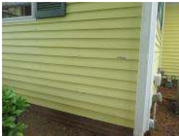
There is significant paint failure and bubbling on the siding and it appears interior spackling was used. Loose and failing paint and spackling will be scraped, sanded, spackled and spot primed as part of the preparation process.
